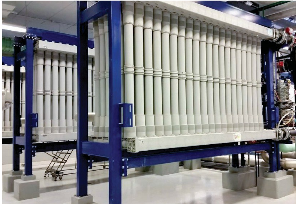
Filters at the BCT Water Treatment Plant
